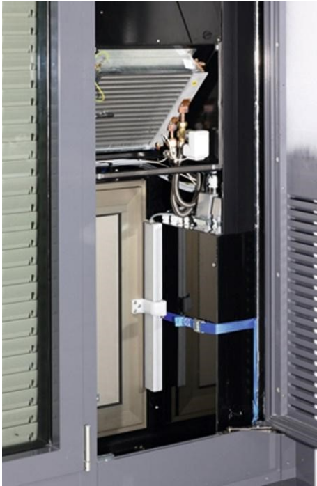
Figure 15: HVAC in TEmotion-Module [122]
