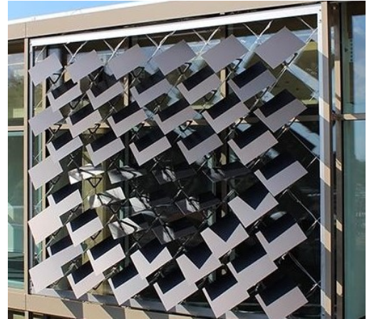
Figure 2: ASF PV-module at HoNR ETH Zürich [33]
